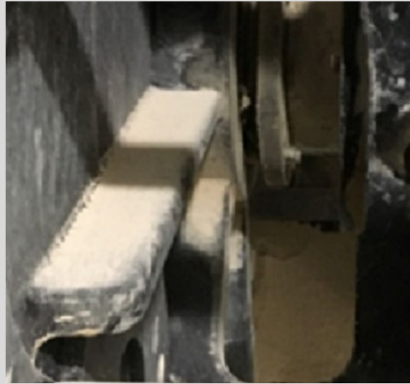
Before: Ash leaking from a rotary feeder
